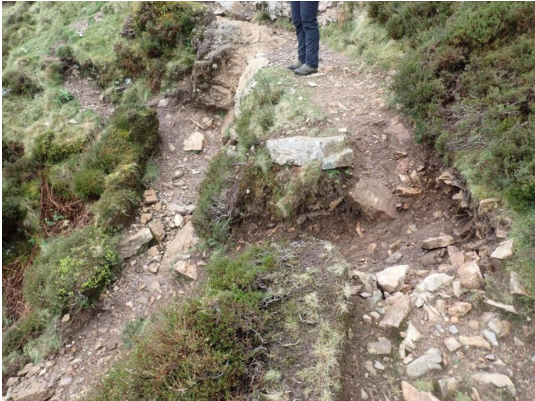
Photo 2 – collapsed revetment with side route joining from below
