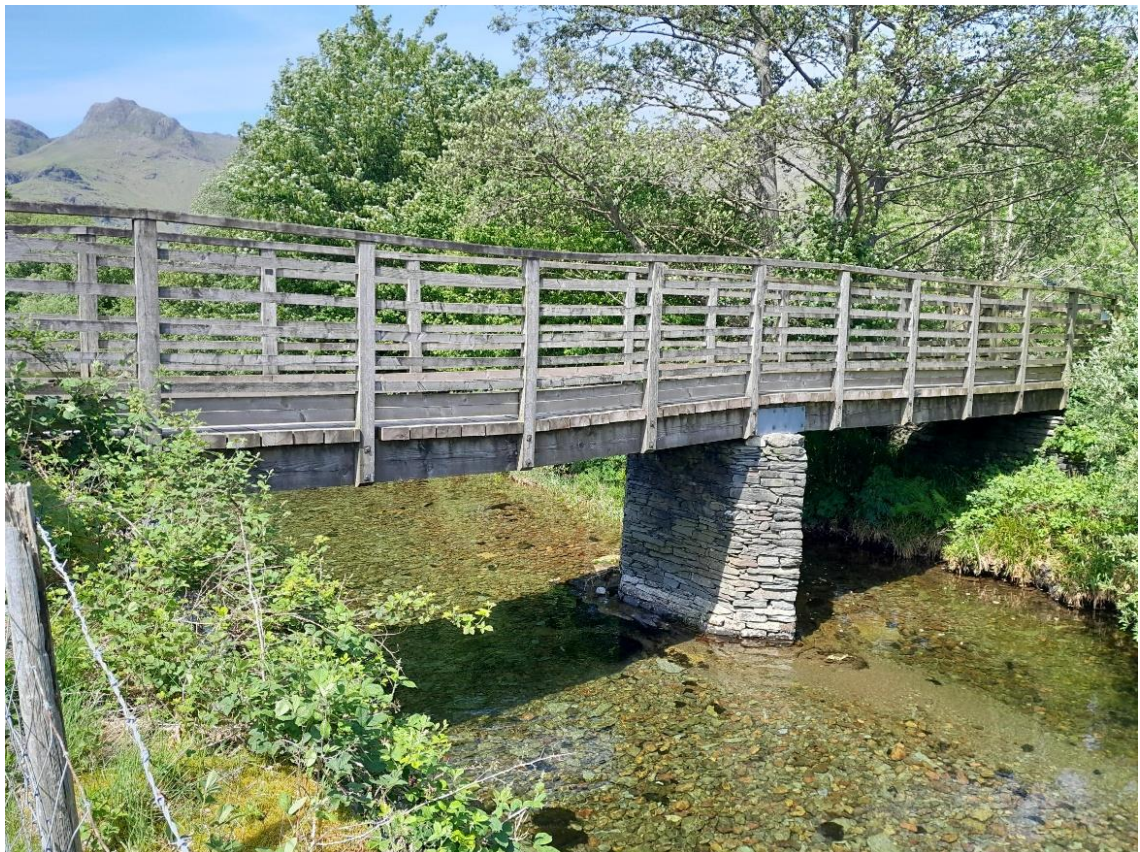
Photo 1 – the beam has visibly deformed
