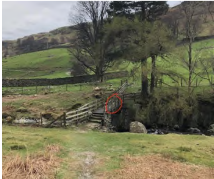
Red circle is from an inspection identifying issue with uprights / handrails
