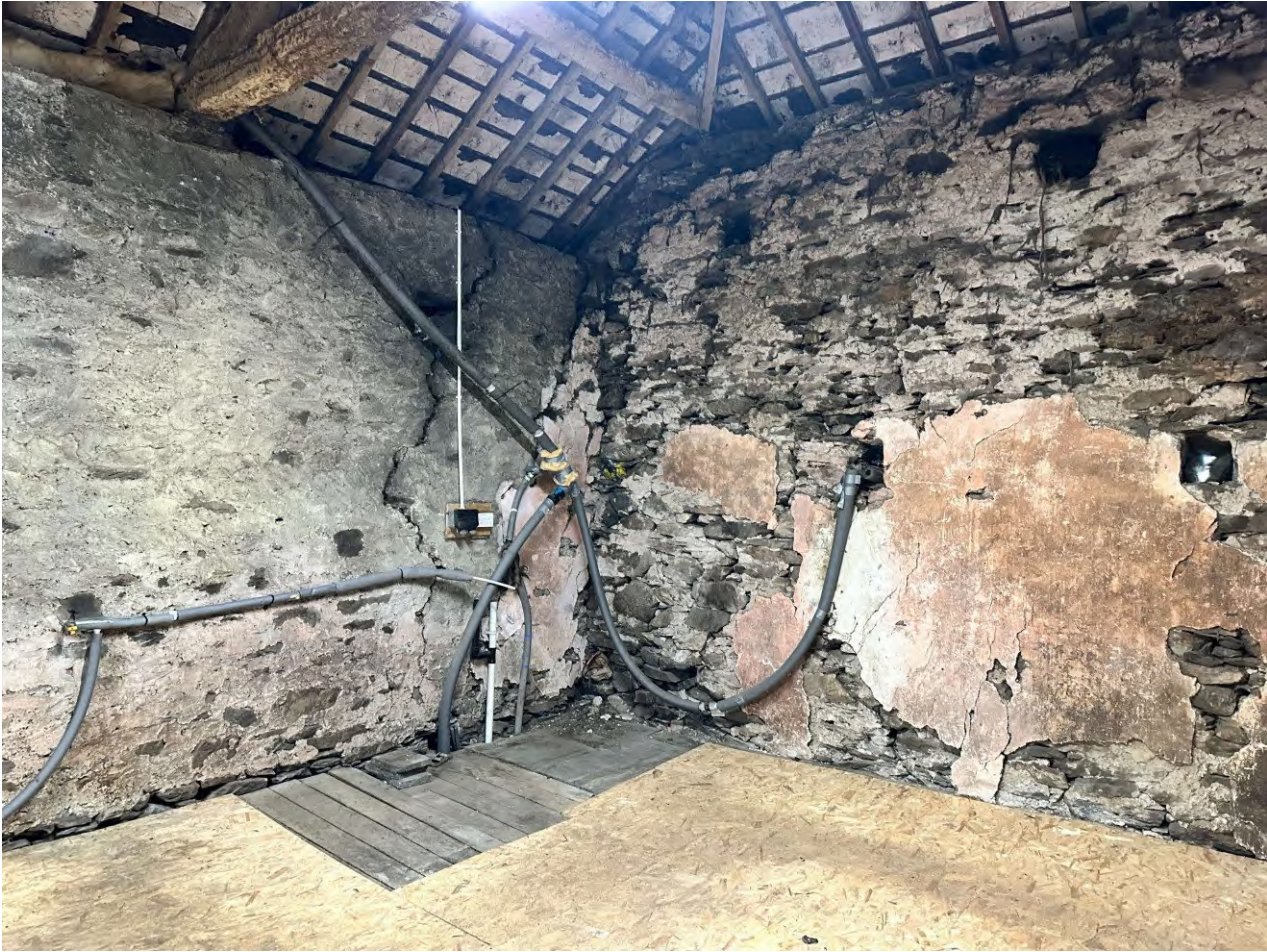
Internal view of the corner of the barn – the crack can again be seen -
