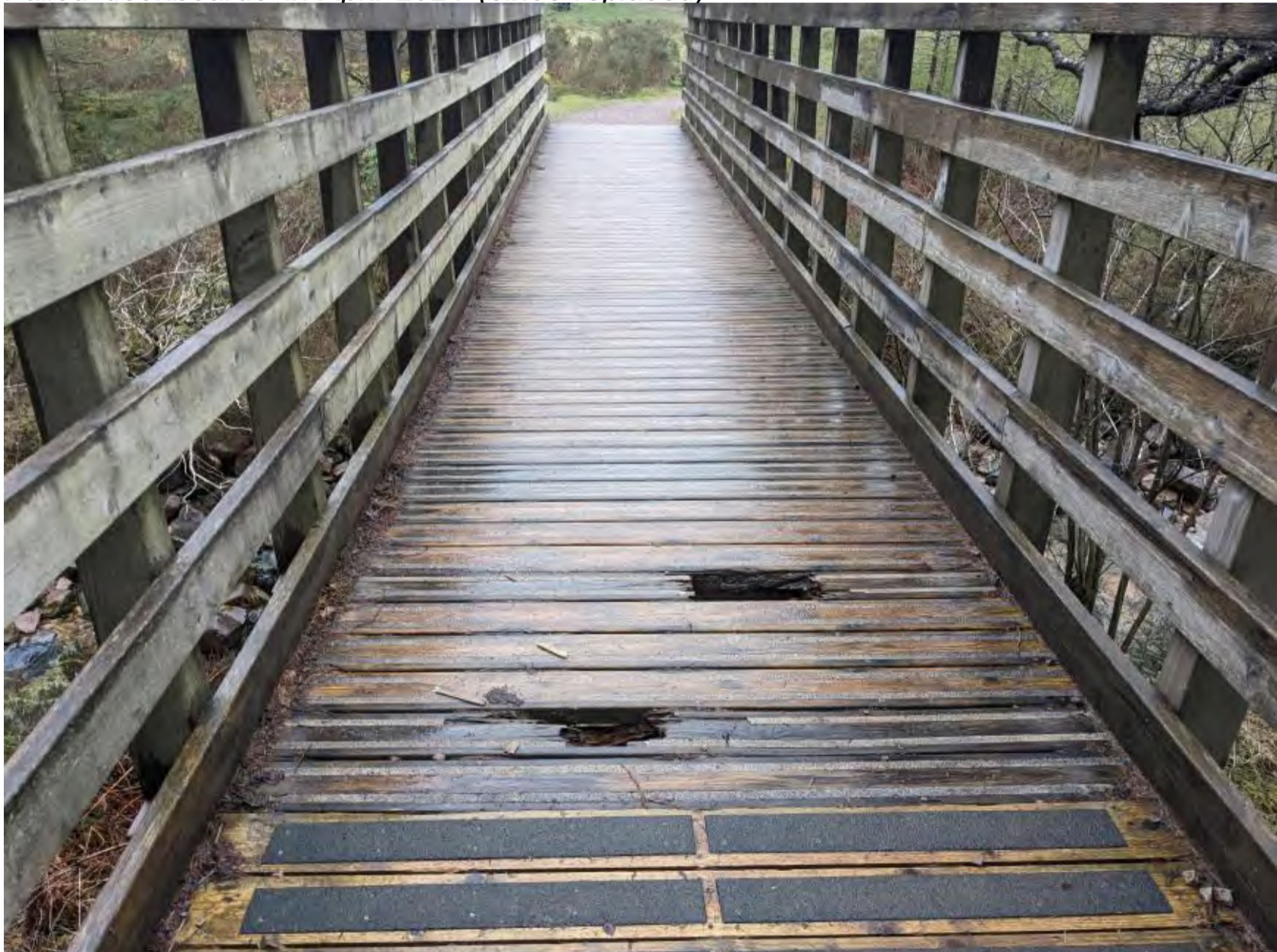
Failed deckboards in April 2024 (since replaced)
