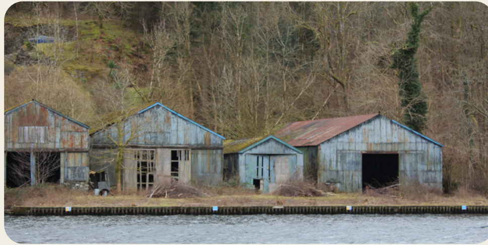
8.3.6 Poor building condition to the south
