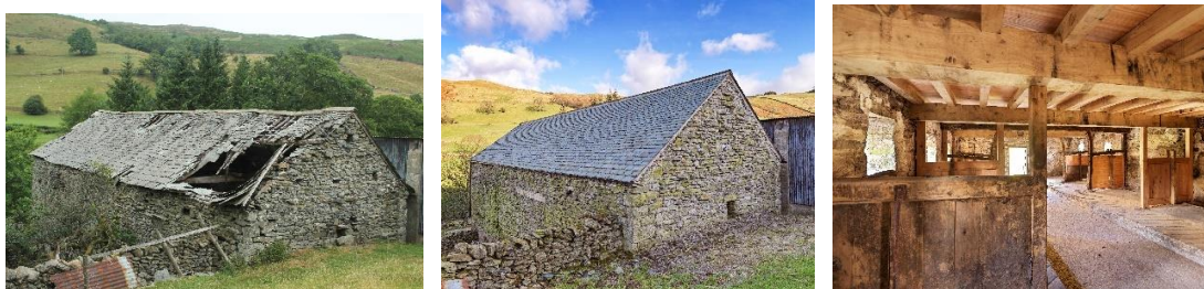
Before and after images of Bridge End Barn, Longsleddale. After images © Historic England – James O. Davies
