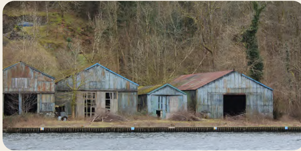
8.3.6 Poor building condition to the south
