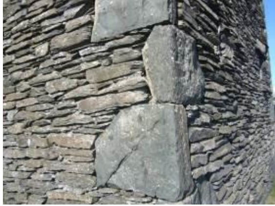
Fig. 13 Roughly hewn large stones make up the quoins of this 18 th century barn.
