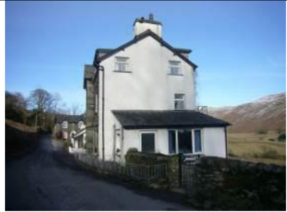
Fig. MP2 This Victorian building has additional flat-roofed dormers, uPVC windows, smooth render and, to the rear, a metal fire escape – none of which are characteristic of the area.
