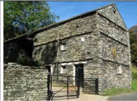
Fig. 3 A typical Cumbrian bank barn at Townend Farm, taking advantage of the slope to access to both lower and upper storeys.
