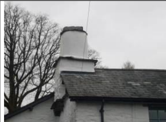
Fig. 43 This chimney has a tapered circular shaft set upon a rectangular base which is cantilevered on short wooden beams.
