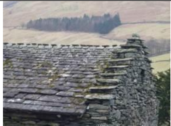
Fig. 44 Crow- or corbie-steps are the names given to a distinctive stepped projection of the gable-end wall above the level of the stone slates. Note also the ridge of 'wrestler' slates.
