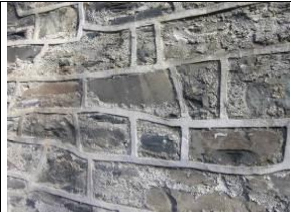
Fig. MP6 An example of inappropriate re-pointing of stonework which is unsightly and possibly damaging to the stone.
