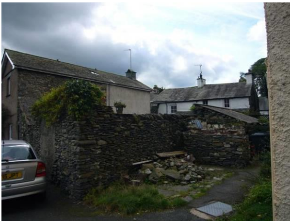
Buildings and outhouses at risk on Back Lane
