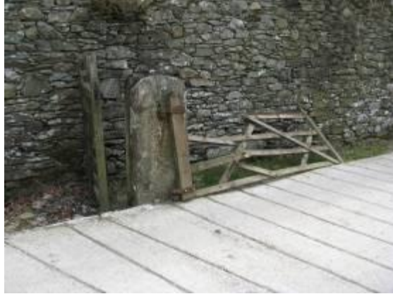
While the general condition of structures within the conservation is good, there are some features that require repair and maintenance.
