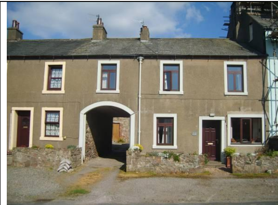
Fig MP1 This house has modern windows and the lower right-hand window opening has been enlarged.
