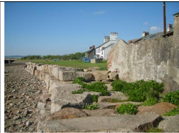
Fig 1 Sea wall that forms part of Ravenglass flood defences at The Green.
