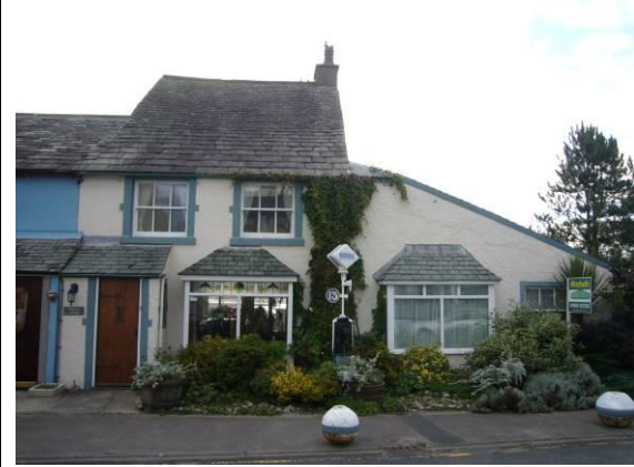
Fig 33 Roof of slates laid in diminishing courses, i.e. large ones at eaves, small ones at ridge.
