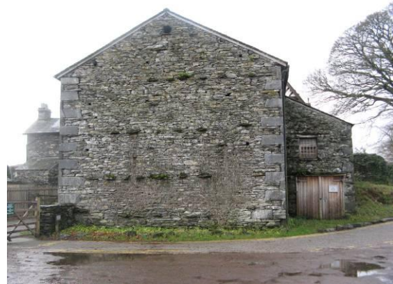
The bank barn (Saw Mill) is constructed of limestone and features distinctive 'through stones'.
