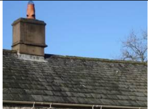
Fig. 10 Slate roofs are laid in diminishing courses i.e. small slates at the ridge graduating to large slates at the eaves.
