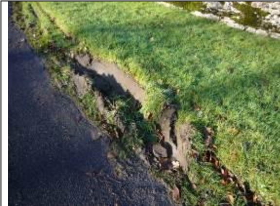
Fig. MP3 Grass verge eroded by passing vehicles.
