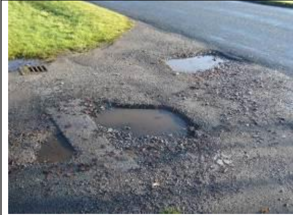
Fig. MP1 Access road in need of repair.
