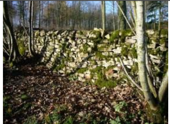
Fig. MP4 Stone wall in need of maintenance.
