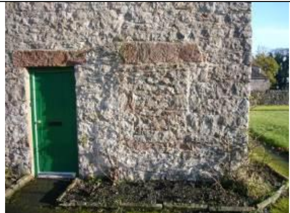
Fig. 28 Blocked opening to the right of the door. The cottages have been altered over the years, most notably in the 1960s.
