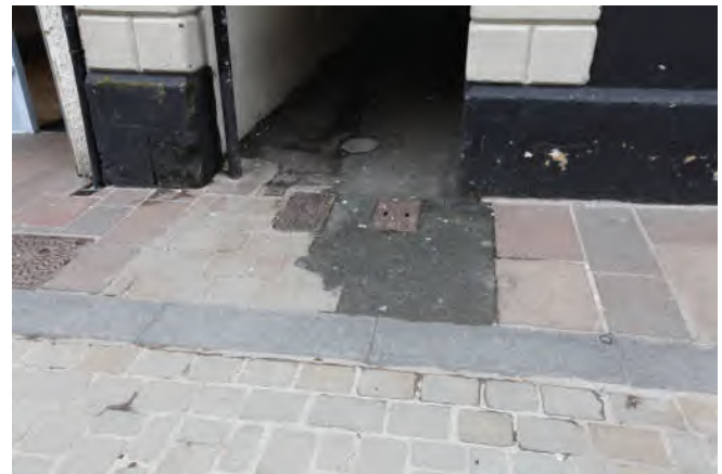
13.48 Publicly funded pedestrianisation scheme with patch repairs in blacktop. Trench works to repair a service have caused this problem.
