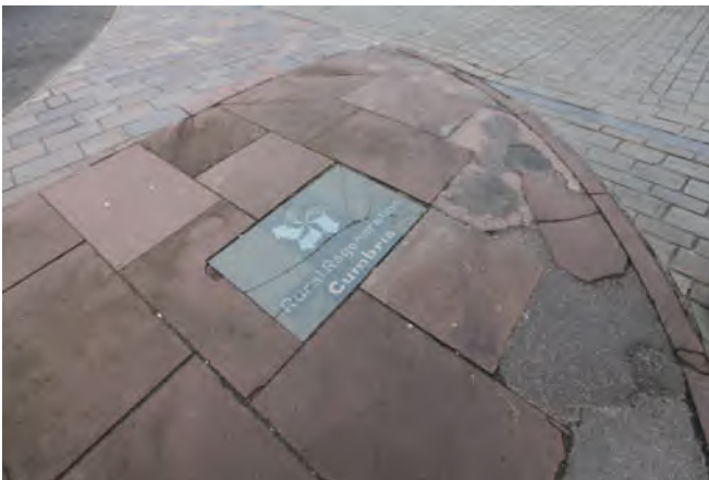
13.47 Publicly funded restoration scheme with patch repair and broken flags. Vehicle over-run has caused this problem.
