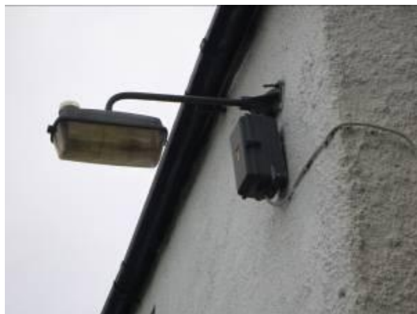
Fig. 14 Simple functional wall-hung street lighting
