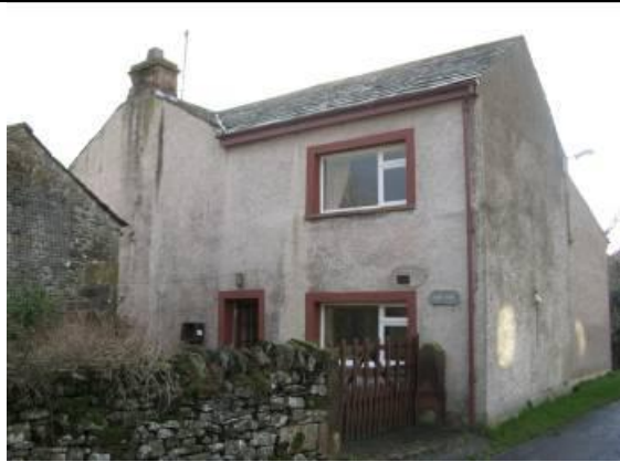
Replacement windows which do not follow a traditional glazing pattern are detrimental to the character of a historic building.
