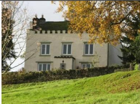
UPVC windows at Castle Villa are detrimental to the character and appearance of historic buildings.
