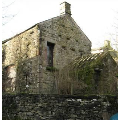
Some structures in the conservation area are in poor condition.
