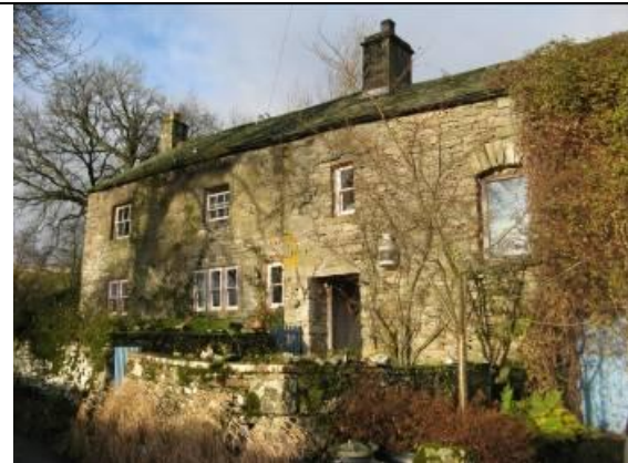
The farmhouse at Fell Gate Farm is a rare example of an un-rendered domestic building.
