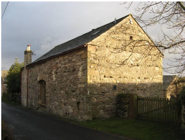
Fig. 3: This barn at Low Side Farm is one of the many agricultural buildings scattered throughout the settlement. The building is constructed from limestone rubble with 'throughstones' on the gable wall.
