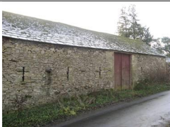
This single storey barn has a large cartshed entrance and vertical slit ventilation holes.
