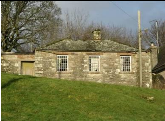
The former school house fronting the green is in poor condition.
