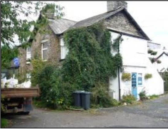
Building at risk from lack of maintenance.
