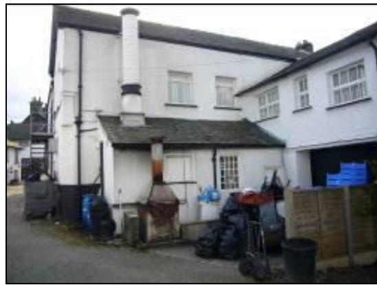
Intrusive extractor vents, gas canisters, refuse containers and fire escapes on a grade-II listed building.
