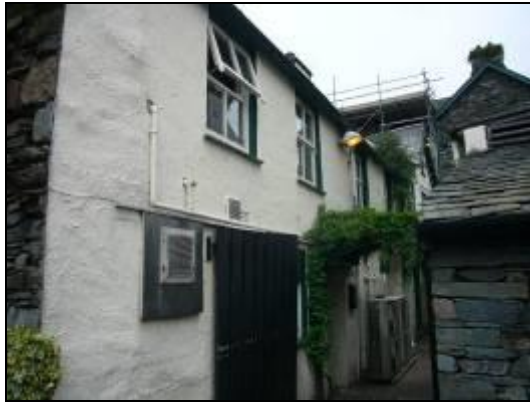
Air conditioning systems, extractor fans and uPVC replacement windows in what is a Grade-II Listed building.
