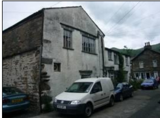
Despite being listed, this former barn has suffered from inappropriate repointing and the application of a modern render coat, which is now stained with damp mould. Replacement windows, overhead wires, the extractor fan and the intrusive waste pipes add to the buildings distressed condition.
