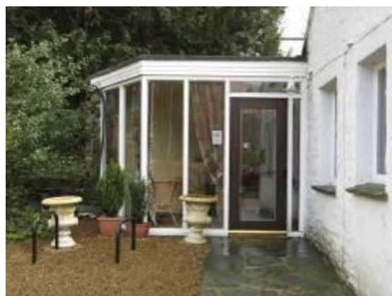
Inappropriate modern materials used in extensions can erode the character and appearance of the conservation area.
