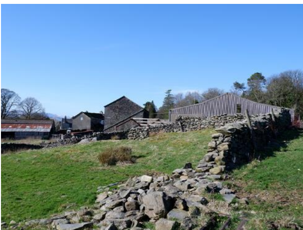
A damaged traditional dry stone wall on a farm.
