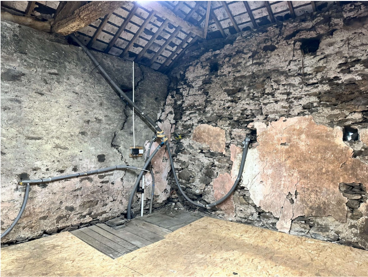
Internal view of the corner of the barn – the crack can again be seen -
