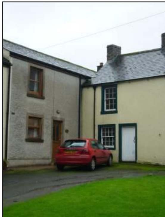
Fig 29: Showing the difference between inappropriate modern materials (left) and traditional ones (right)
