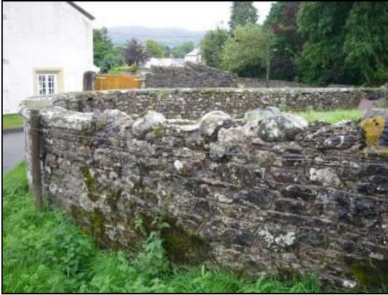
Fig. 14: This wall at Nettle Syke marks the transition from rubble field wall (right) to the more formal coped wall of quarried stone that leads to the entrance gate of the farm
