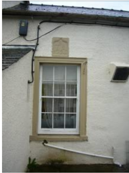
Fig 31 Wires, pipes and extractor fans can diminish the character of rare historical detailing.
