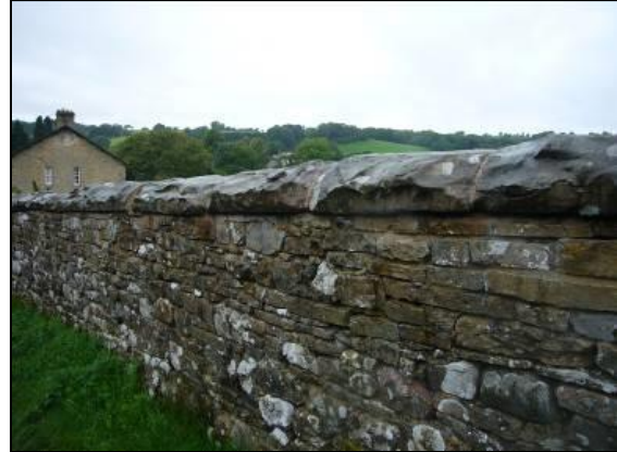
Fig 15: Walls topped by water-worn slabs quarried from a river bed near the Old Brewery
