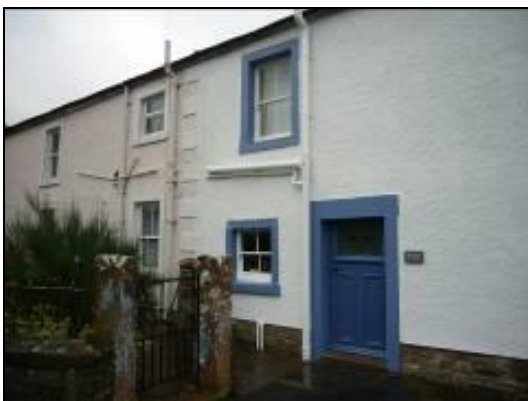
The siting of water and drainage pipes can have an impact on the character of historic buildings
