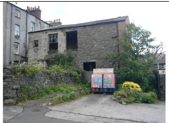
Fig. MP8 This building in Market Street is in need of repair and is an eyesore (Sept 2010).
