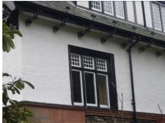
Fig.MP6 Architectural detail such as period windows and ornate metal gutter brackets could be protected with an Article 4 direction.
