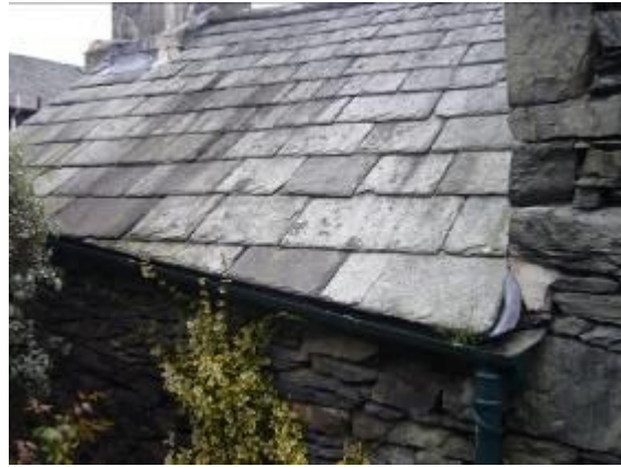
Fig.30 Local stone slates, graded and cut carefully to fill an awkwardly shaped roof.
