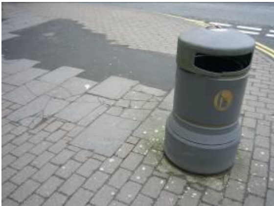
Fig. 40 Pavement surface patched and repatched.
