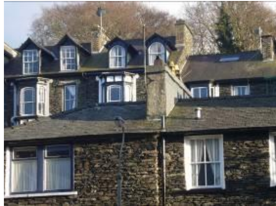
Fig.8 View of rooftop dormers and bay windows in the north-east of the conservation area.
