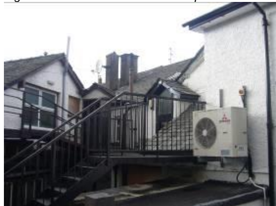
Fig. 43 External fire escapes and air conditioning equipment can be unsightly.
