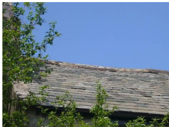
Fig. 36 A roof of graduated greenslate with the smallest sized slates at the ridge.
