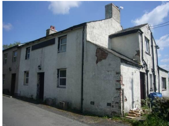
Fig. MP4 The former Moota Inn is in need of remedial works (June 2010).
