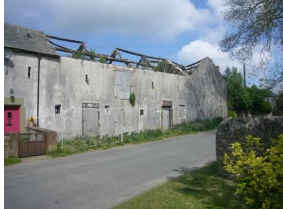
Fig. MP8 The barn at Low Farm is at risk of further decay and in urgent need of attention.
