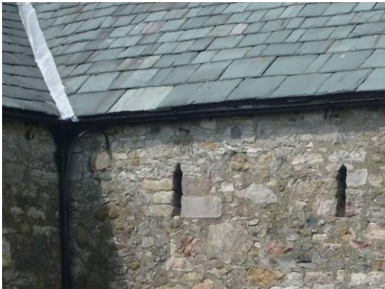
Fig. 37 Typical vernacular building details at High Farm. Note the large boulder stones in the wall.
