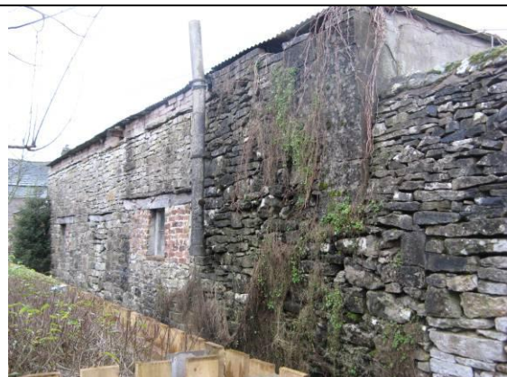
Some of the stone outbuildings in the village require repair and maintenance.
