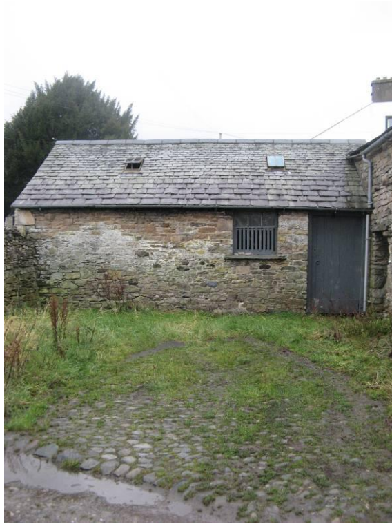
Fig. 7: The narrow back lanes are a distinctive feature of the conservation area and access a number of historic farm buildings
