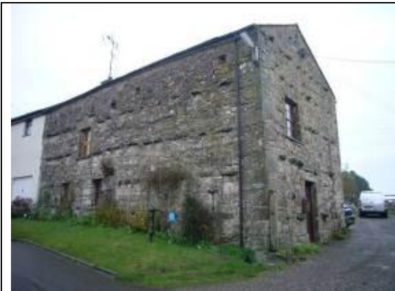
Fig. 37 Whiteside Barn displays characteristic vernacular projecting 'throughstones' that bind the wall together.
