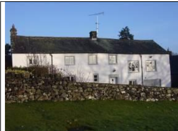
Fig. MP3 Loss of historic detail, including glazing bars, original doors.
