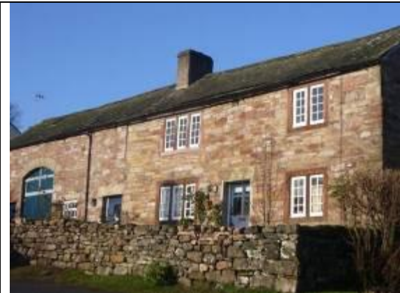
Fig. 19 Stone boundary walls are characteristic of the conservation area – both as field boundaries and garden walls.
