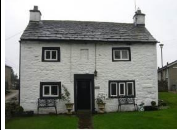
Fig. 9 Small vernacular dwelling with painted rubblestone walls and stone slate roof laid in diminishing courses (large slates at eaves level).
