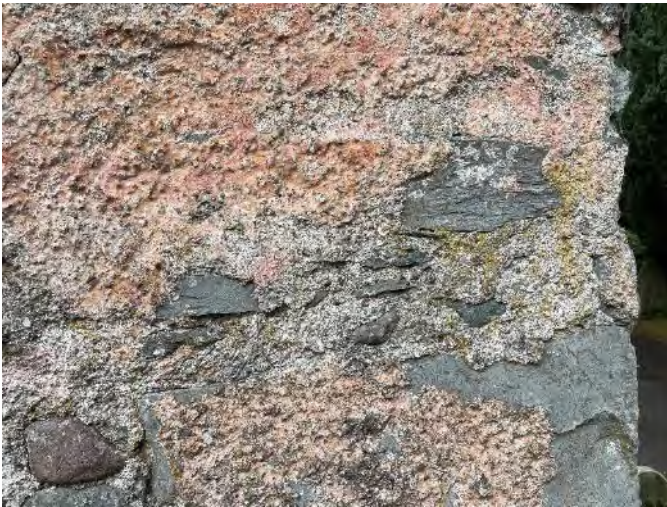
Local stone was often traditionally covered with layers of limewash, as this decaying historic example shows.
