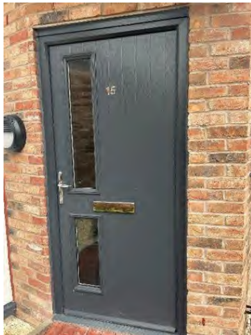
uPVC and composite doors have limited scope for repair or upgrade and must therefore be replaced as soon as they fail or look tired and old. This is a much less sustainable option.
