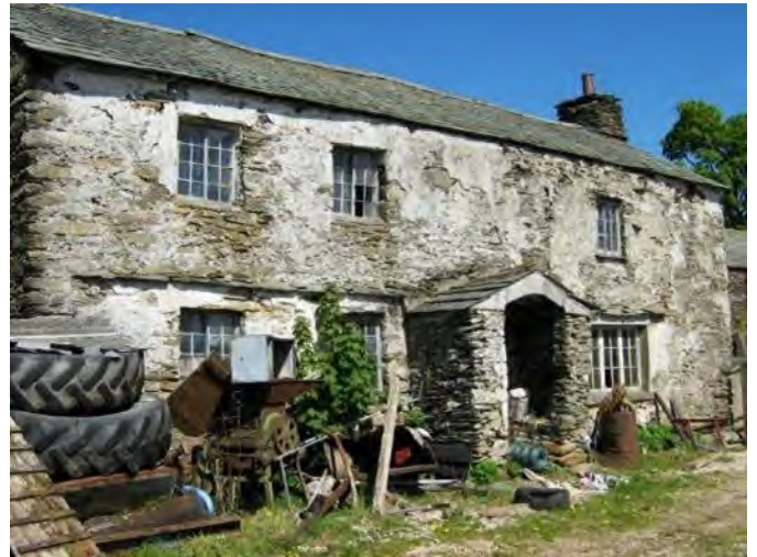
If left to weather, the local stone beneath the render becomes exposed.
