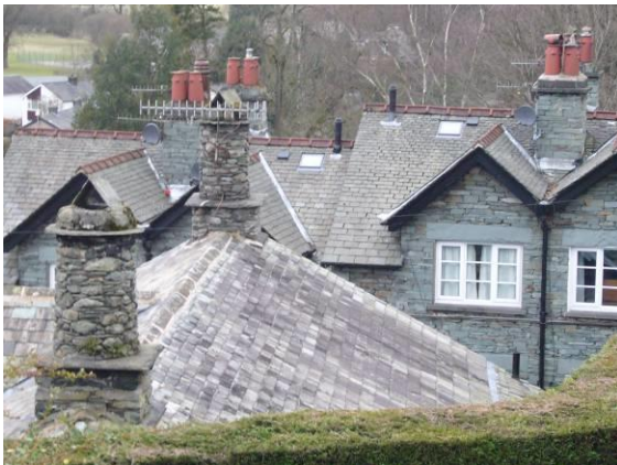
Fig. 5 Part of Ambleside's lively roofscape of stone chimneystacks, clay pots, gables and ridge tiles.
