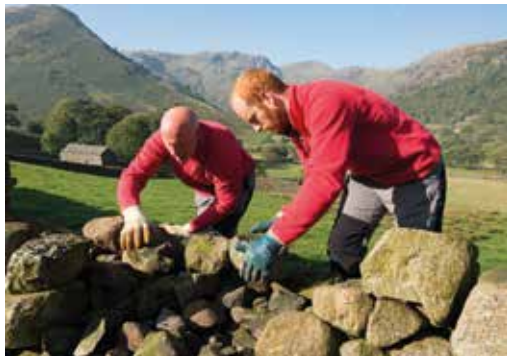
FIGURE 3.10 National Trust staff repairing a stone wall near Hartsop in the Ullswater valley. Stone walling is a traditional skill much prized by farmers and necessary in order to maintain the functionality of the agro-pastoral landscape.
