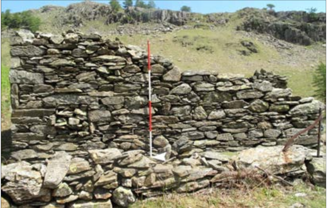
Plate 19: wall 110 of building 100, from the west, showing blocked window 111. In the foreground is boundary wall 801.
