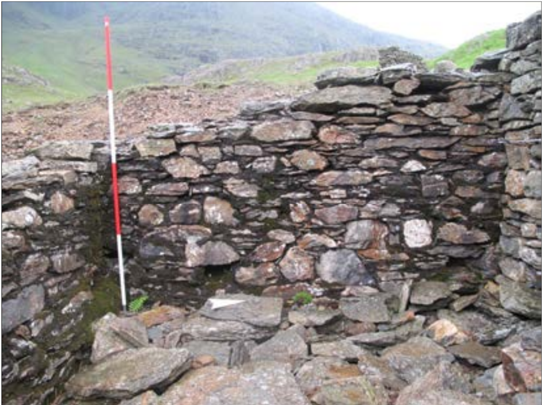
Plate 23: building 200; wall 235 showing voids (235).
