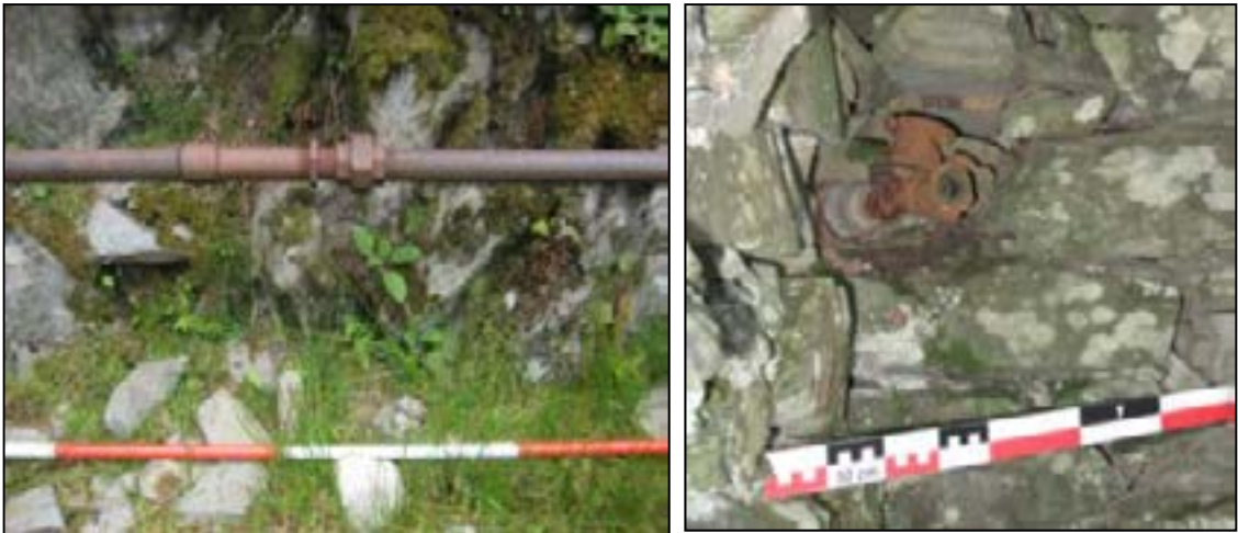
Plates 15,16: (left) compressed air pipe (105), (right) compressed air pipe valve (204) in the smithy
