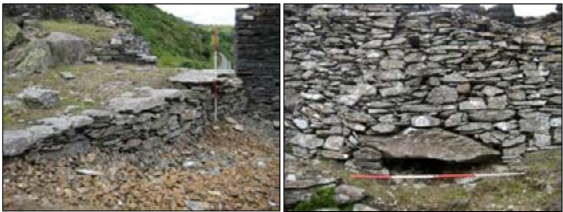
Plates 23, 24: (left) short section of retaining wall (419), covered by later ridge tip at its south end; this may be associated with the mill sorting area and culvert beneath track (420) (right), potentially carrying waste from the ore cleaning operations
