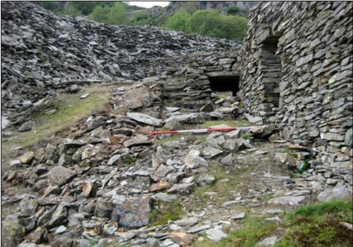
Plate 35: looking west along the exterior of the south wall (507) of the dressing mill. The rectangular platform in this location (approximately the same width as the ranging rod) may be the backfilled remains of a smaller wheel pit associated with the mill
