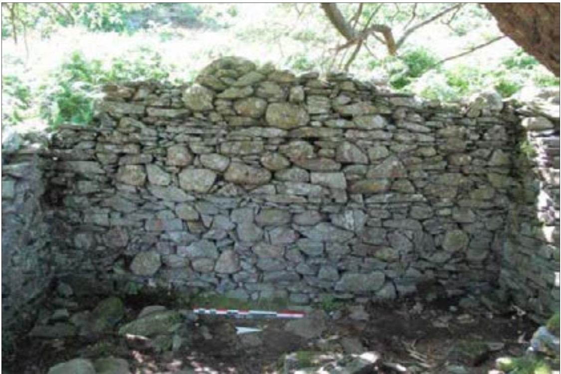
Plate 9: east-facing elevation of smithy back wall (205) showing the levelling of the wall at intervals with smaller flat pieces of slate
