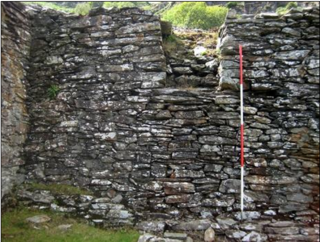
Plates 36: angled recess (504) in wall (501); one of two chutes for tipping crushed ore from the crusher into the dressing mill
