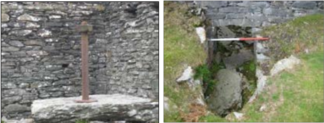
Plates 29, 30: (left) detail of one of the holding bolts at the top of the wheel pit (320) and (right) vent of race at the base of wheel pit (303)
