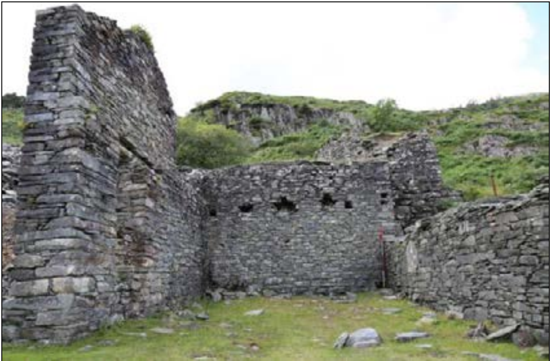
Plate 31: east-facing wall of the crusher house (401), with first floor joist holes (402). The ground floor void (405) can be seen at the base of the vertical ranging rod
