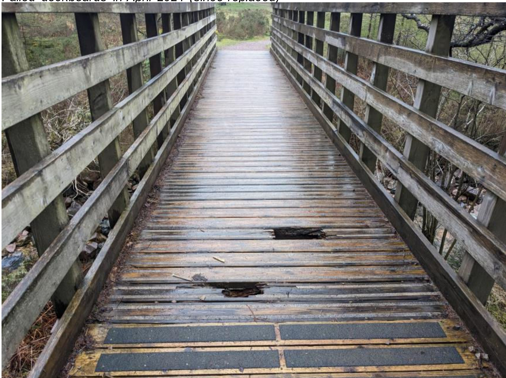
Failed deckboards in April 2024 (since replaced)
