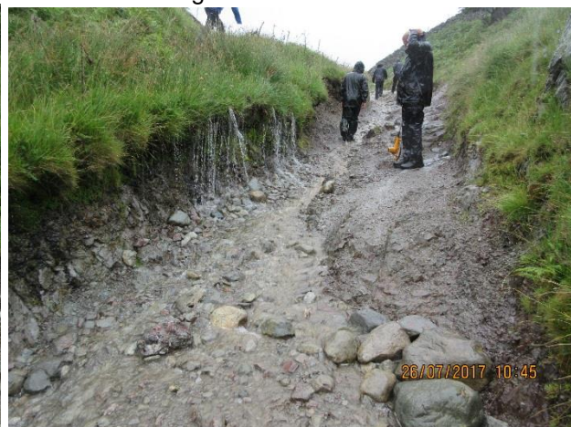
4: Looking up, old drains on left, water not being collected
