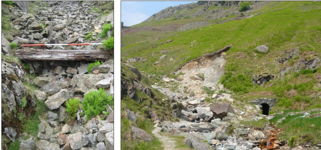
Plates 54 & 55: problems with erosion. The first is Middle Level, blocked by fallen scree and spoil, the second is bank erosion along Red Dell Beck, just above the entrance to Deep Level.
