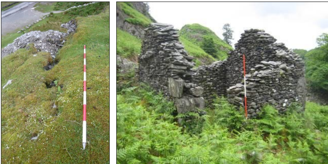
Plates 50 & 51: crack along the north-eastern edge of the main rid tip at Penny Rigg Quarry and bracken growth surrounding the powder magazine (2042) and weakening the stonework over time.
