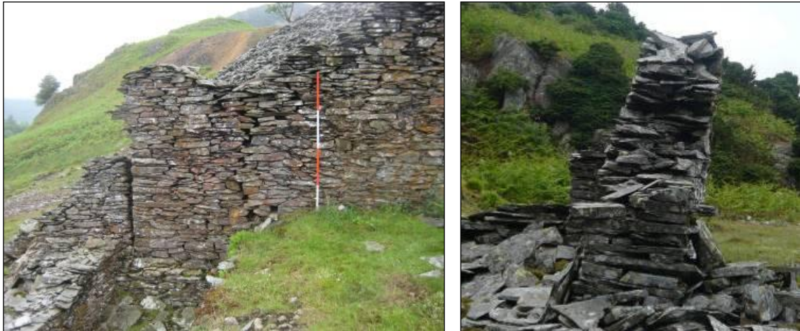
Plates 48 & 49: severe cracking in the wall of the (2051) and leaning gable wall in danger of imminent collapse on building (2072) at the old quarry (2071).
