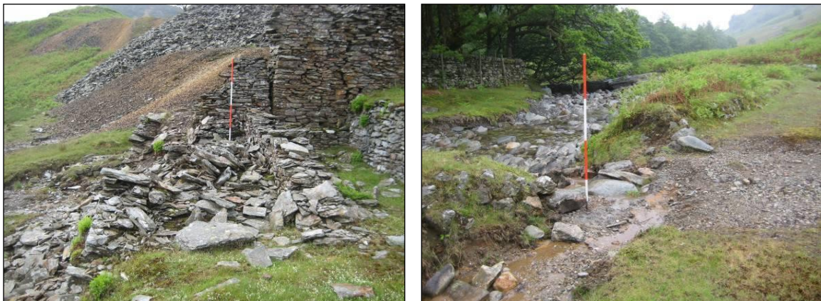
Plates 52 & 53: flood damage winter 2009/10 – damage to Dressing Mill (2051) and erosion along the Yewdale beck, potential washing contaminated soil into the river.
