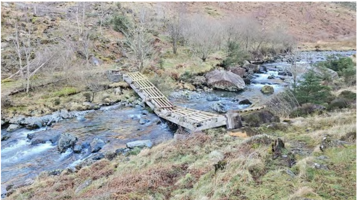
Photo provided by LDNPA volunteer of the damaged bridge
