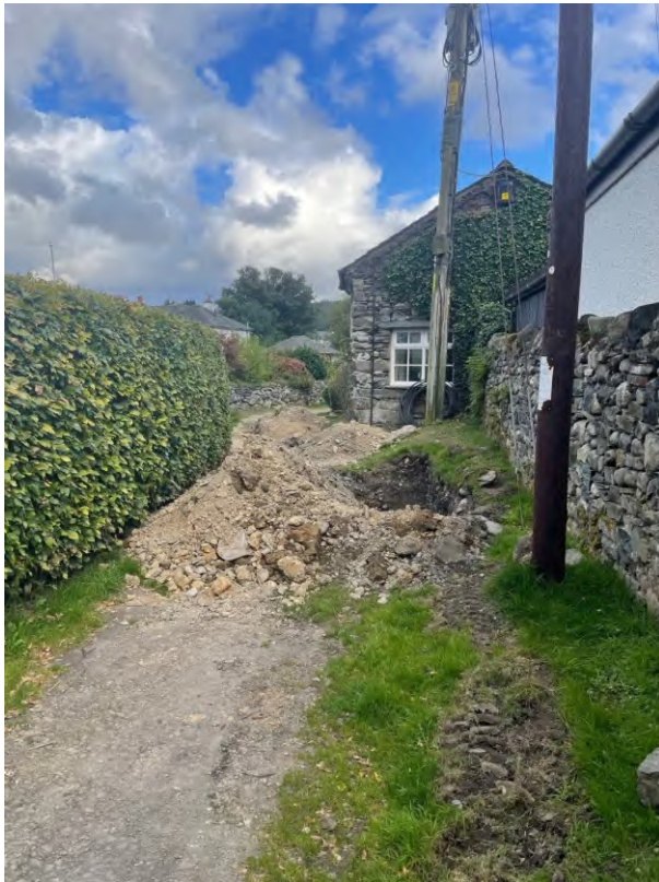
Excavation of path surface and rotten electricity pole leaning
