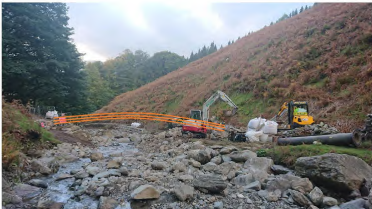
Photo 3: Location of new flood-resilient bridge over Greenhead Gill (point D on map below).
