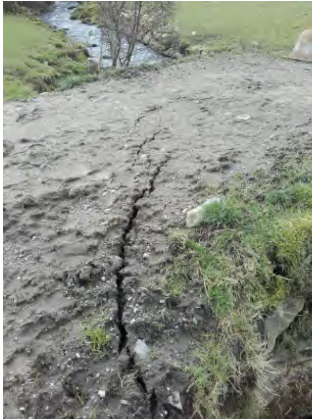
Crack in surface has appeared
