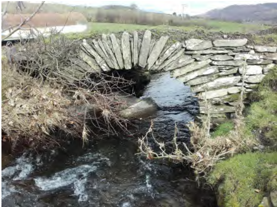
Photo of bridge – the stones in the beck are from the arc on the upstream side, and a hole has developed by the left abutment – some slippage can be seen on the right side of the bridge arch
