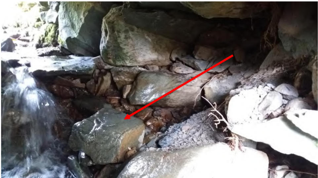
Photo of abutment showing slipped stone(s)
