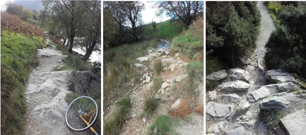
Some of the sections between D & F that are currently difficult to use.
